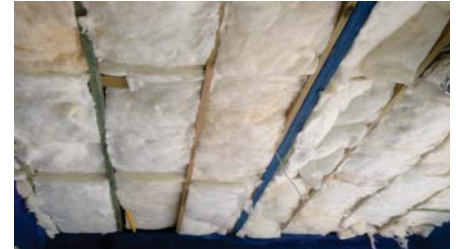
* Formaldehyde Free Glass Wool Insulation installed in residential ceiling
